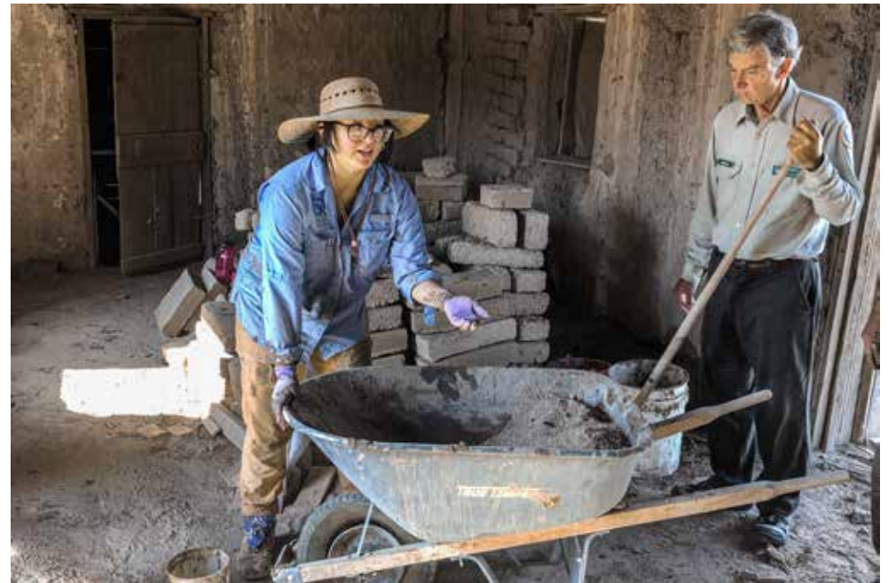
Big Bend Conservancy teamed up with the National Park Foundation and the Center for Big Bend Studies at Sul Ross State University to restore adobe work at the historic Alvino house in the Castolon area.
